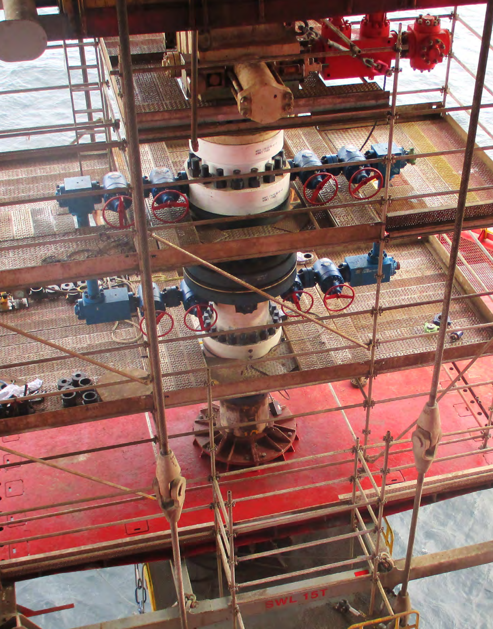
POS-GRIP 20k Wellhead System for Total Solaris X-HPHT Well
